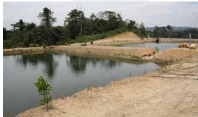
[GAM] Newly created settling reservoir
