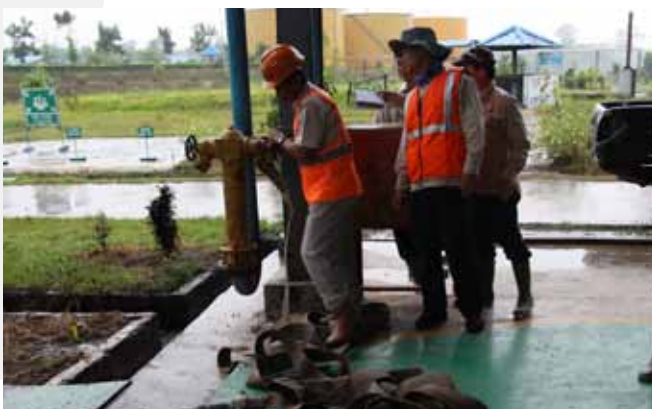
[Palm] Checking drills for fire and emergency cases at CPO Mill
