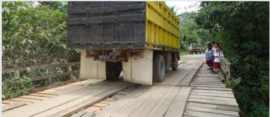
Existing decrepit wooden bridge
