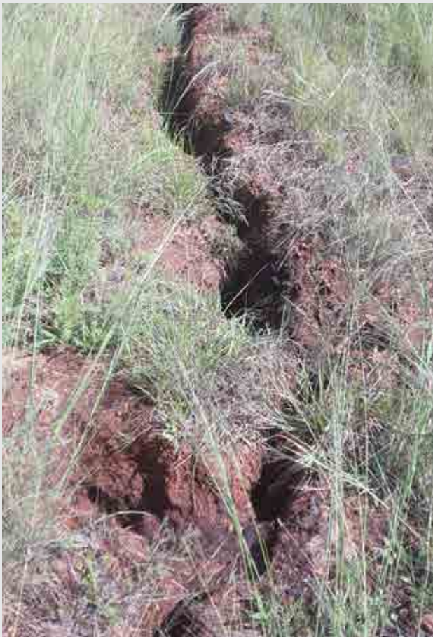
Figure 2: Some of the cracks caused by differential settlement
