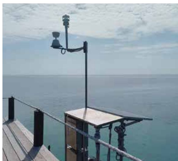
Marine Telemetry Station
