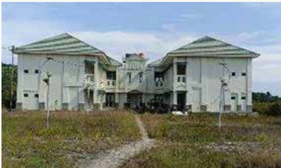
Condition of the STAIS (Sekolah Tinggi Agama Islam Sangatta/Sangatta Islamic College) building after renovation
