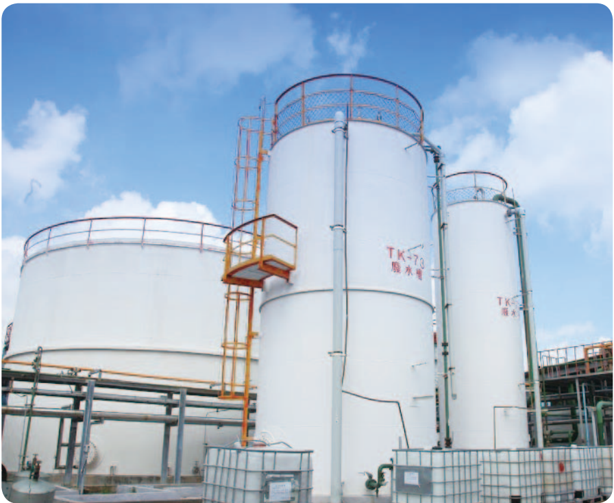
Wastewater processing tank
