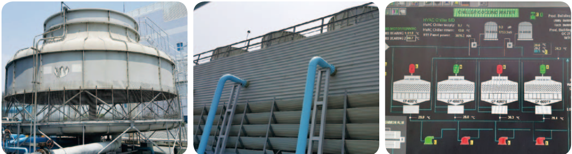
Old cooling tower
