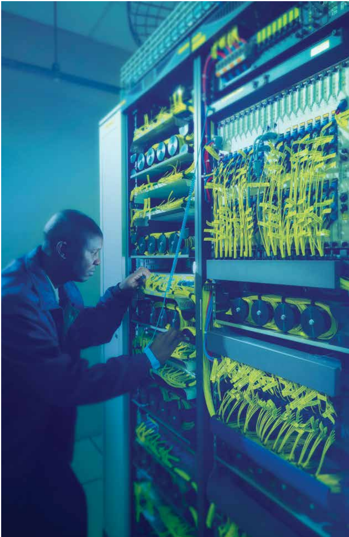
Rack on which fibre to the home technology terminates in the exchange
