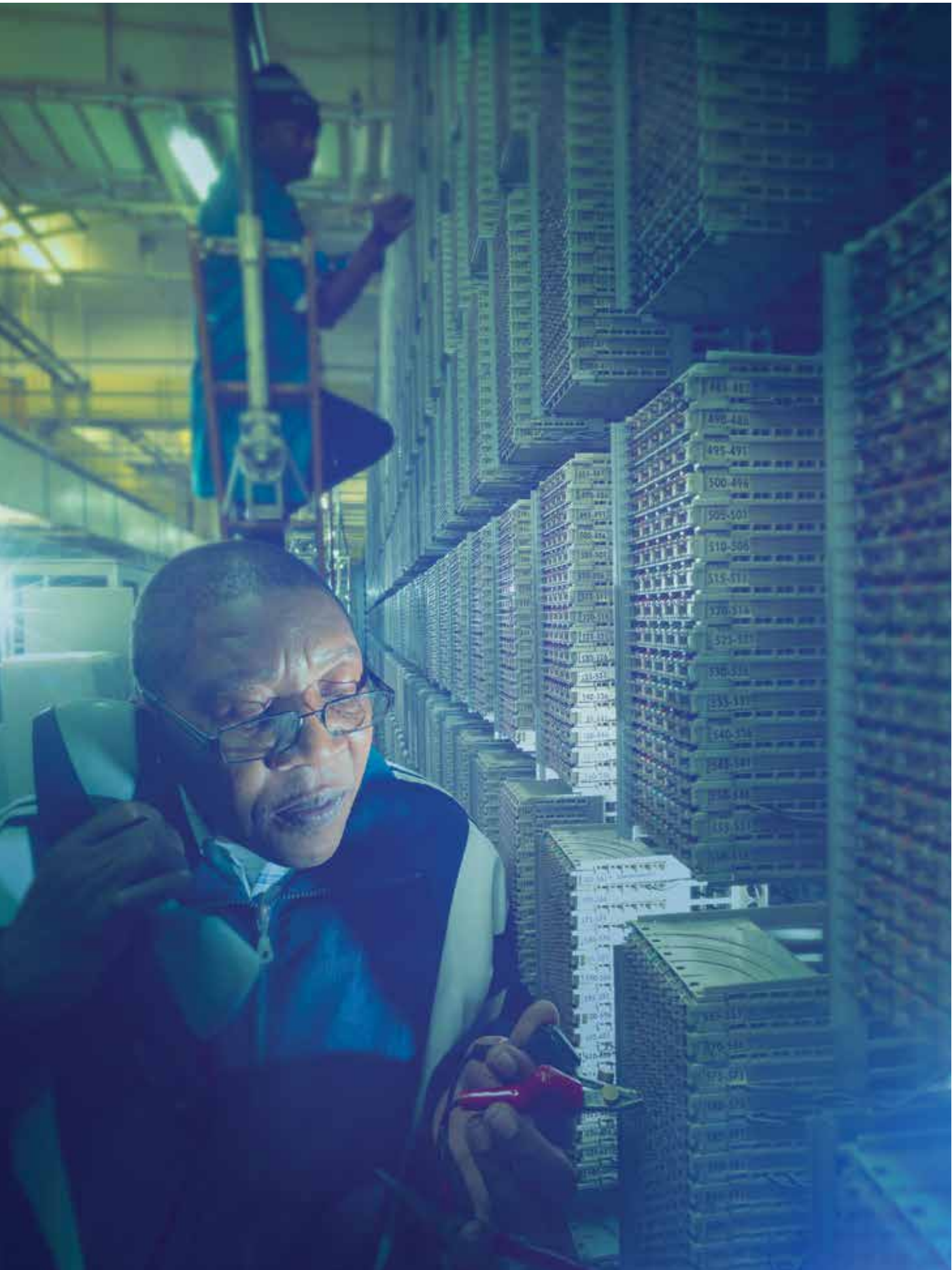
A main distribution frame where copper cables connect between the outside world and the exchange
