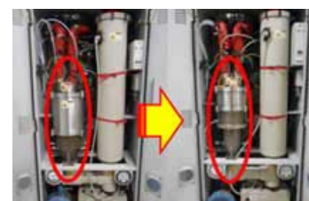
Upgrade exhaust gas treatment furnace on machine stations
