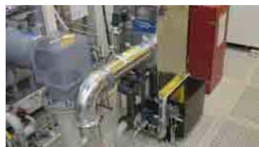
CS IPA Scrubber Discontinued Water Washing
