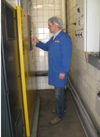
Marc Reckhemke in the operation of the of frequency-controlled compressors.
