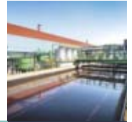
PLANT WATER TREATMENT PLANT
