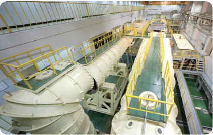
Joint Water Tank
