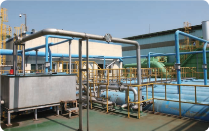
Wastewater Treatment Plant (Geoje Shipyard)
